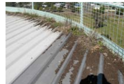
Kick rail ponding
