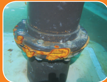
New ductile iron pipework corroding.
