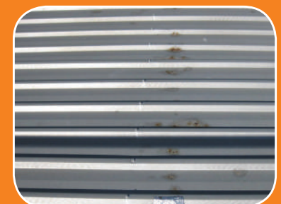
Roof sheet corrosion from safety mesh below.
