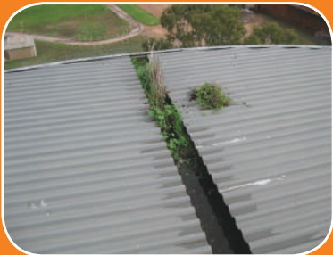
Box gutter blocked and overflowing.
