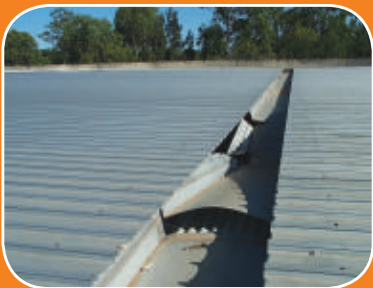
Box gutter collapsed.
