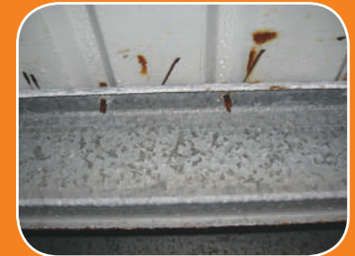
Corroded roof screws and safety mesh.
