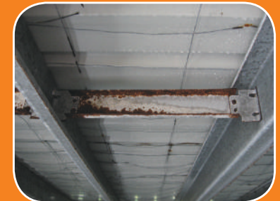
Corroded purlins and safety mesh.
