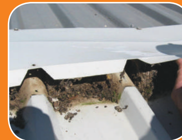
Ridge capping debris.
