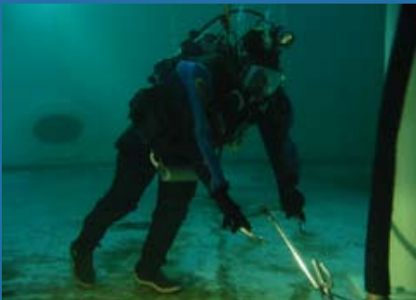
The Aqualift vacuum system
