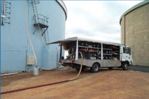
Aqualift pumping system
