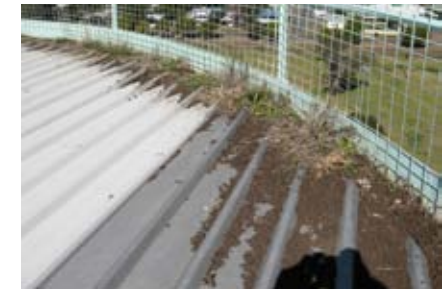
Kick rail ponding
